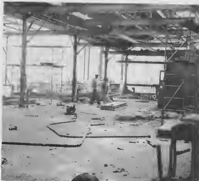
In a scene reminiscent of the Korean War, two workmen dismantle the old welding shop (12). The structure of this building, plus the old carpenter and pipe shops will go to make a 10,600 sq. ft. warehouse space (16). Air conditioned storage will also be added.
